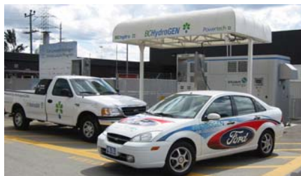
Canada: World First 700 Bar H2 Refueling Station
